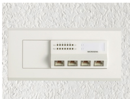
Micro Switch with cover installed in a concealed wall socket
