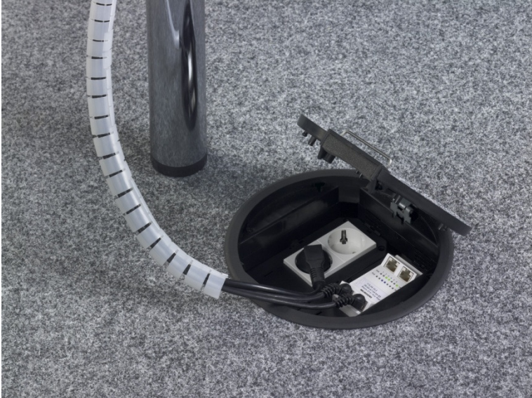
Floor tank (open)
